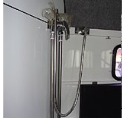
Inbuilt shower at rear inside of float
